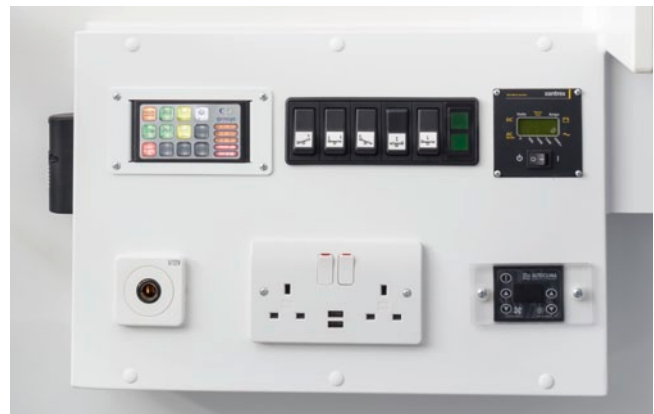
The central operation panel for the control of the electro hydraulic table, AC system and the lighting.
